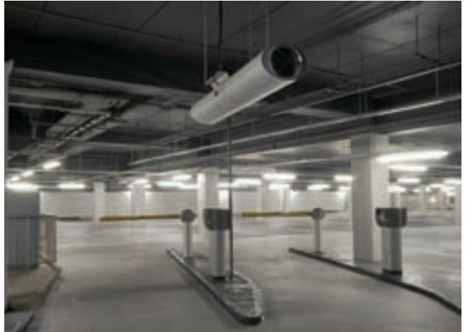
After: Improved ventilation systems, 70% energy savings, less clutter
