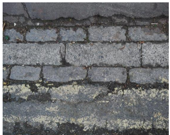
Figure 42 – Granite setts to drainage channel.
