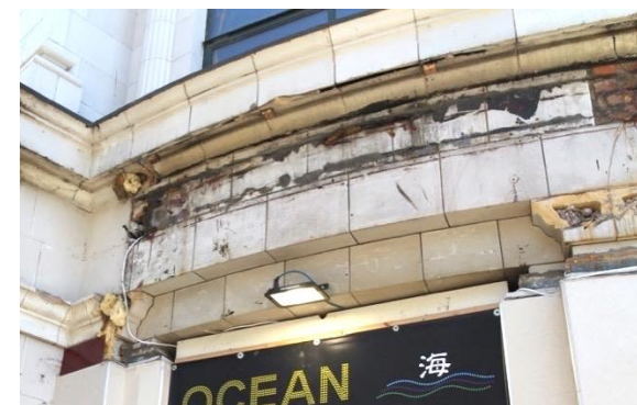
Figure 7 – Loss of cornice and capital white glazed Terracotta to former cinema, East Street.
