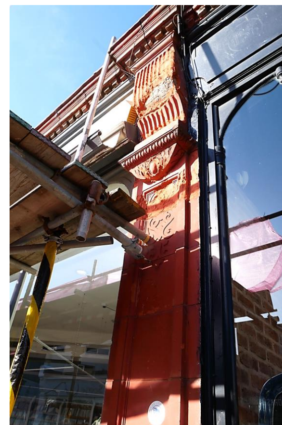
Figure 11 – Terracotta pilaster and corbel eroding but also damaged.
