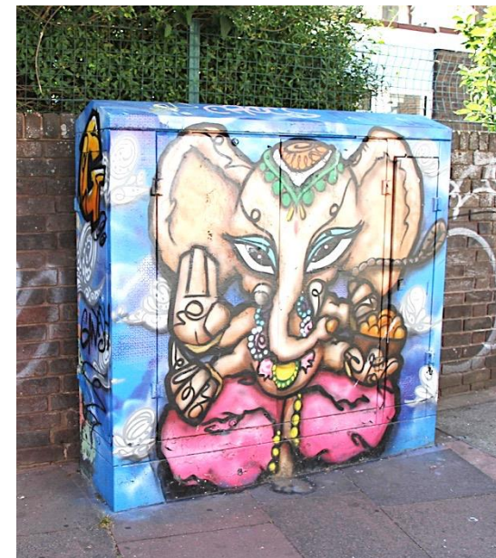
Figure 30 - a graffiti covered utilities cabinet.
