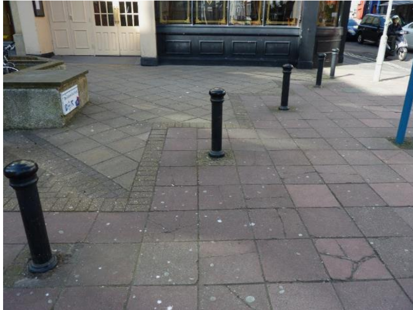
Bartholomew Square: incoherent street surfaces poorly maintained
